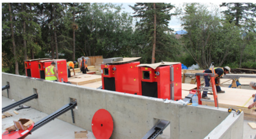
Four of the ten heating systems that will be installed
